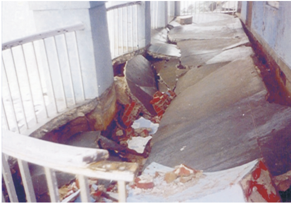
Figure 2. Damage of LeCafe Restaurant due to the Coastal Erosion.
